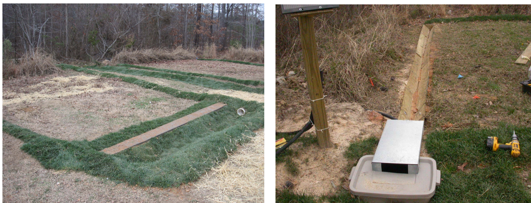
Figure 2. Level spreader, recollection trough, and weir box.
