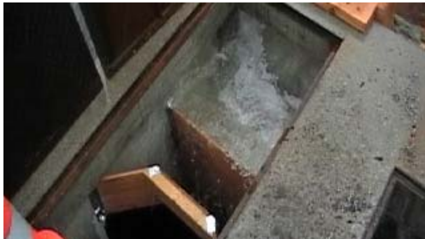
Figure 1. View of Inlet/Outlet Bay and a portion of the StormFilter Bay at 59 l/sec (2.1 cfs), 27 seconds into “instant-on” hydraulic test. Note that StormFilter Bay is still empty which indicates that the system is still in the process of filling.
