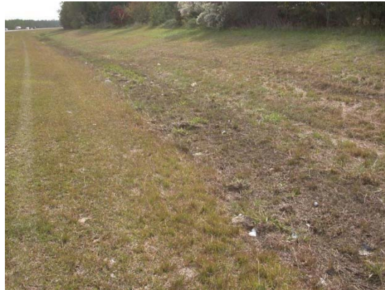
Figure 2 Example of a vegetated swale without wetland characteristics (i.e. standard dry swale).
