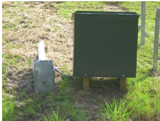
Figure 7. Weir Box for sample collection at edge-of-pavement and VFS outlet.
